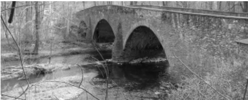
Mortonville Bridge over Strasburg Road is listed on the National Register of Historic Places.
